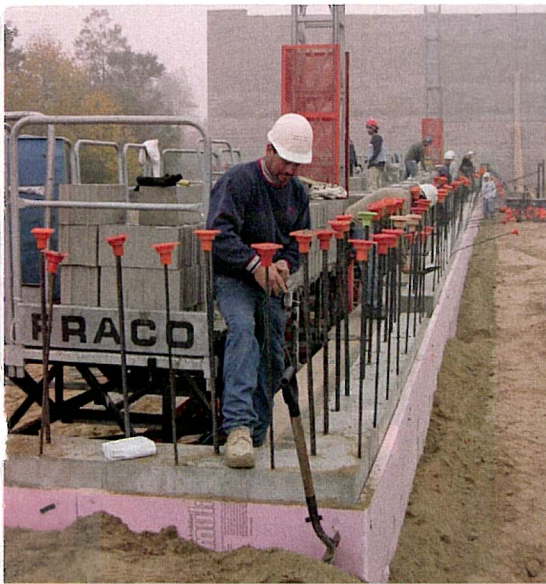
Left: Using Fraco mast-climbing work platform, Pynn Masonry employees prepare to erect CMU load-bearing wall.
